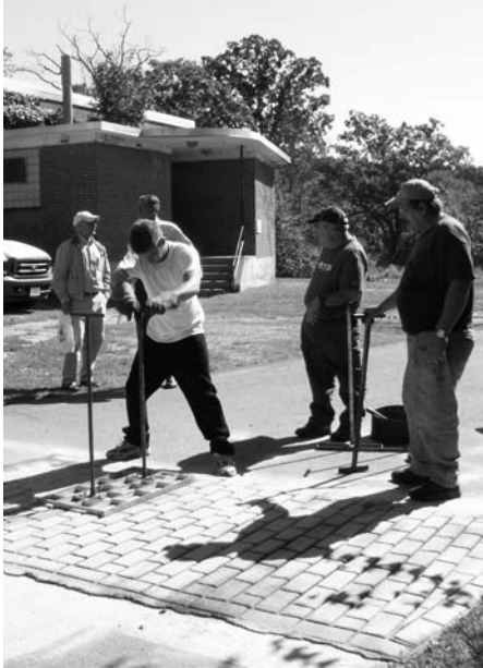
Demonstrations, such as pavement texturizing, allowed participants to view new materials and procedures.
